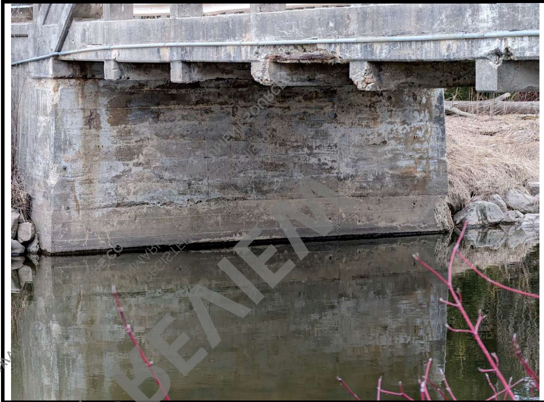
Photo 15 Scaling on foundation of east abutment wall
