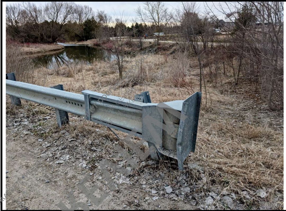
Photo 7 Vehicle damage on northeast end treatment
