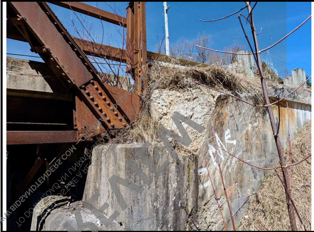
Photo 13 Concrete Disintegration at SE wingwall
