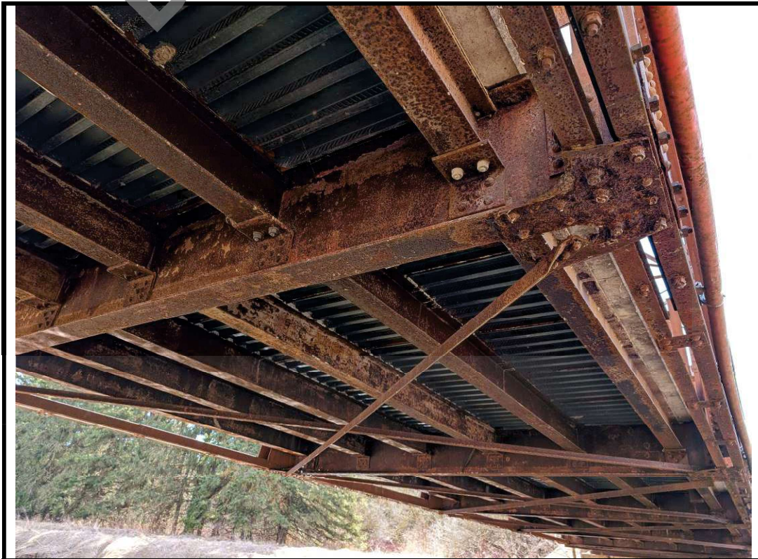
Photo 10 Perforations on north bottom chord
