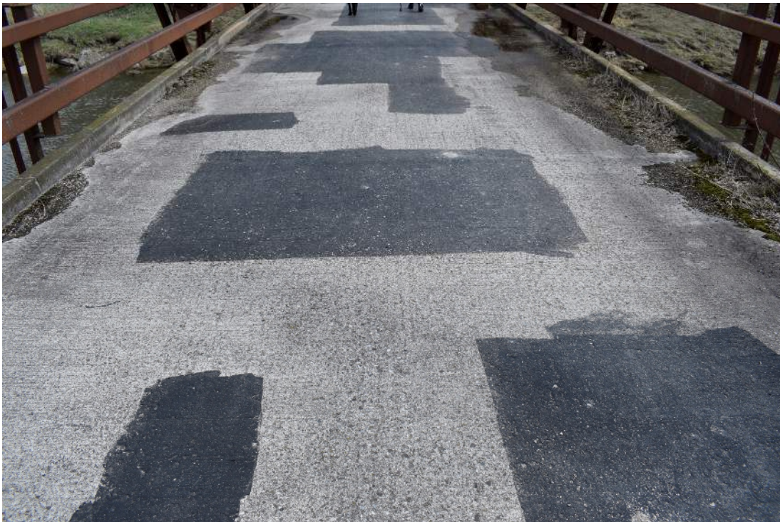
Figure 46: Condition of road surface
