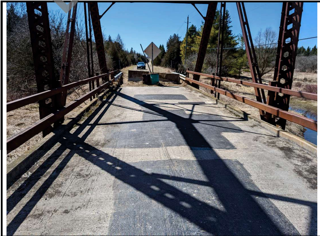
Photo 8 Previous asphalt patches on deck wearing surface
