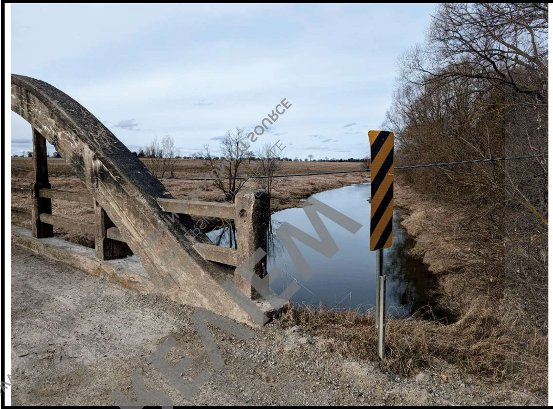
Photo 9 Typical view of southwest hazard sign
