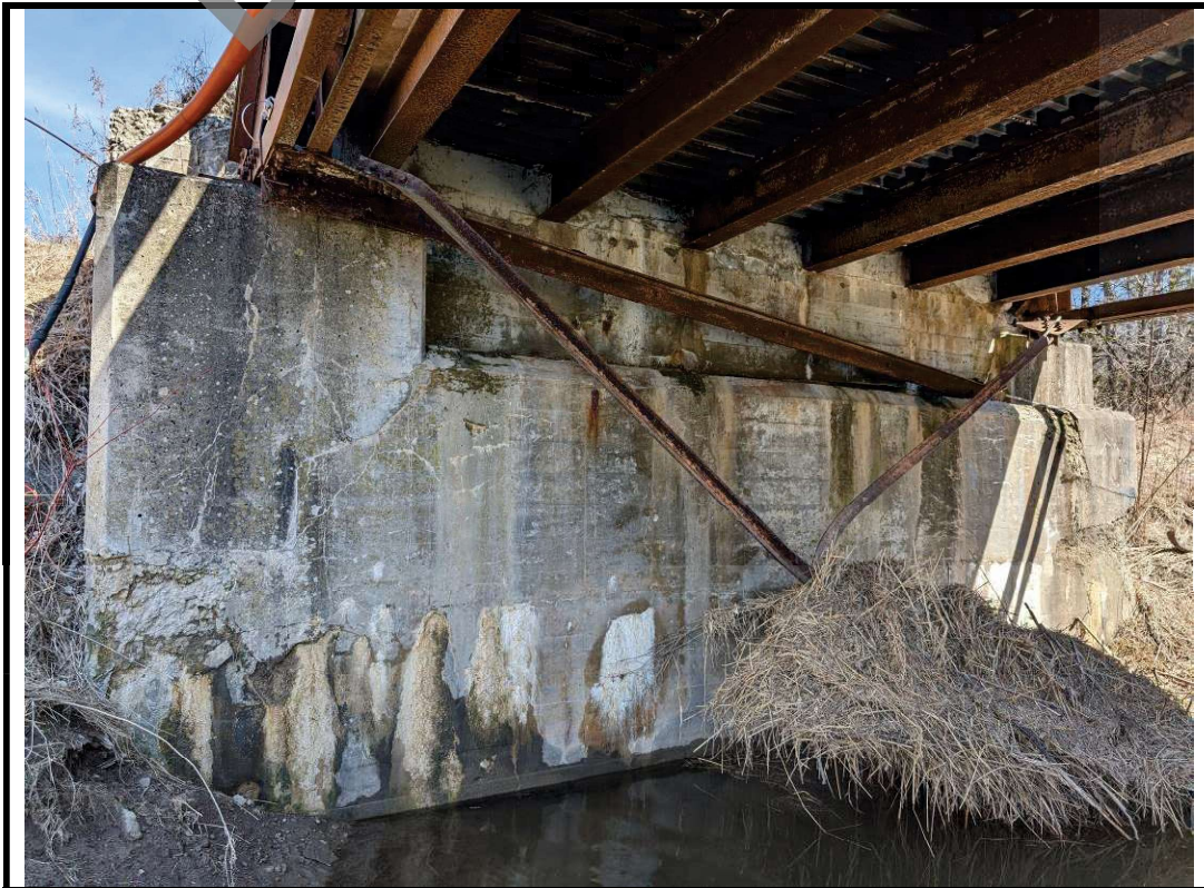
Photo 12 Damaged bracing at east end of structure
