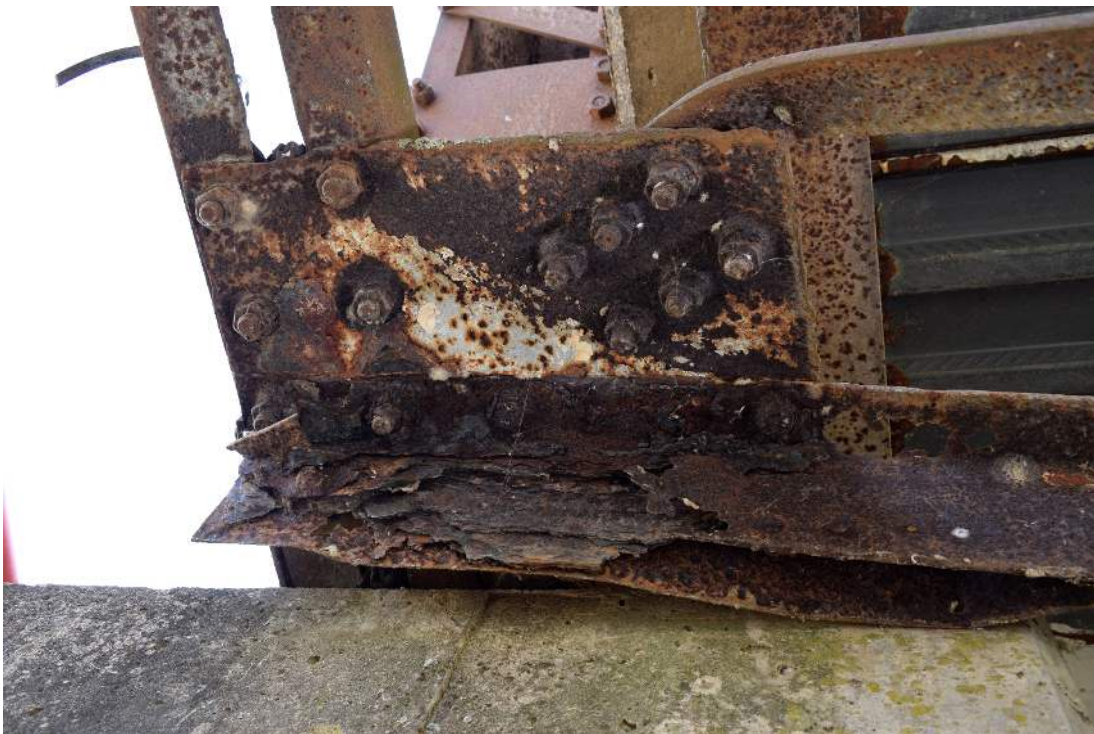
Figure 48: Example of typical deterioration of structural steel
