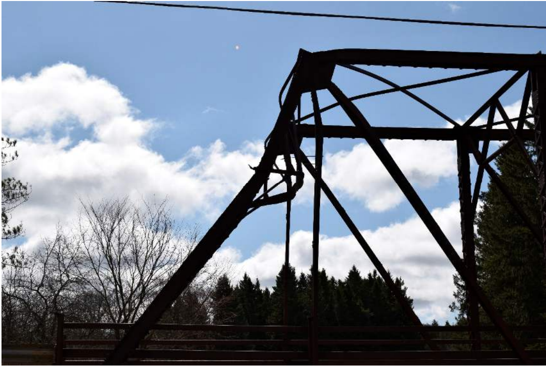
Figure 45: Side view of west end damage
