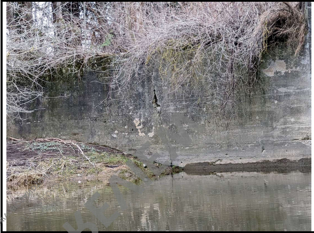
Photo 21 Vertical wide crack on southwest wingwall
