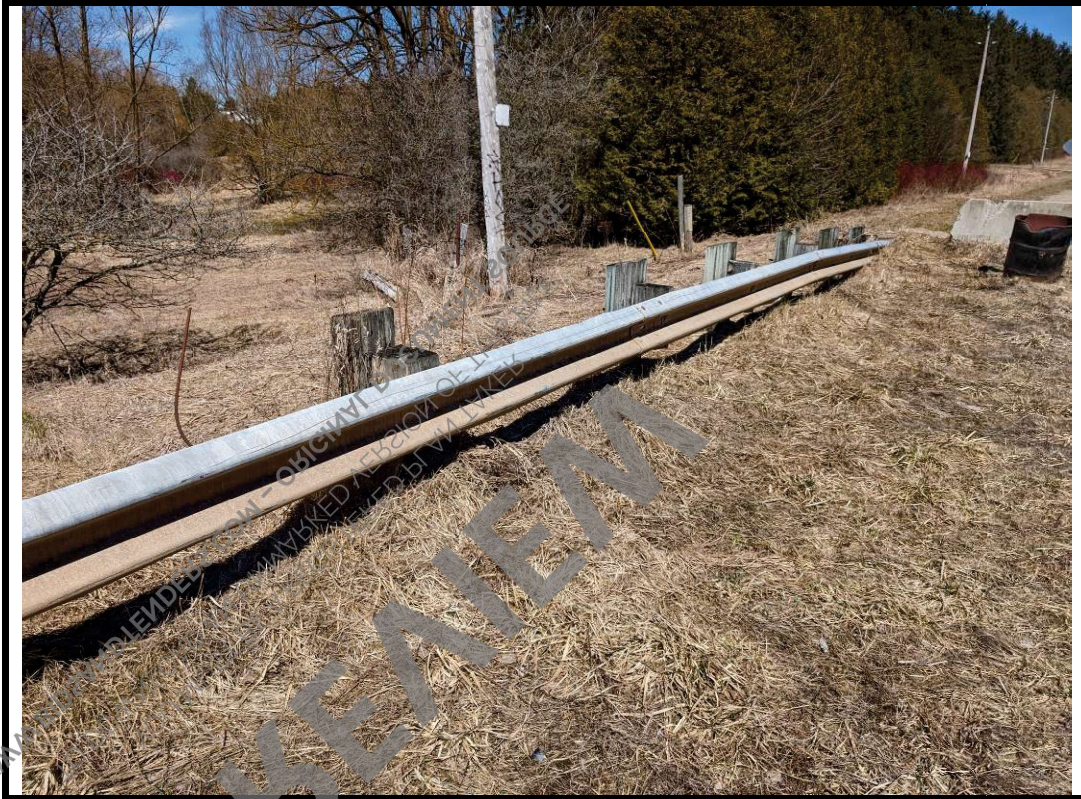
Photo 7 Substandard approach barrier at NE approach
