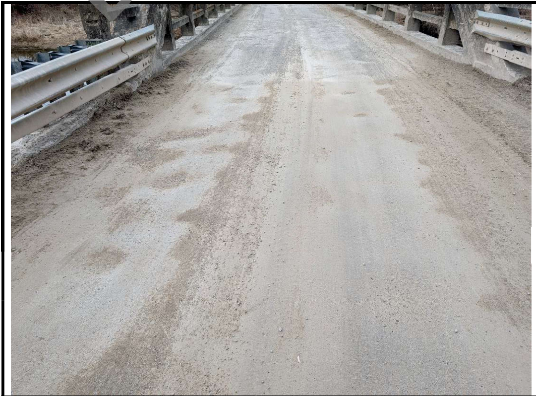
Photo 8 Potholes on west approach near deck
