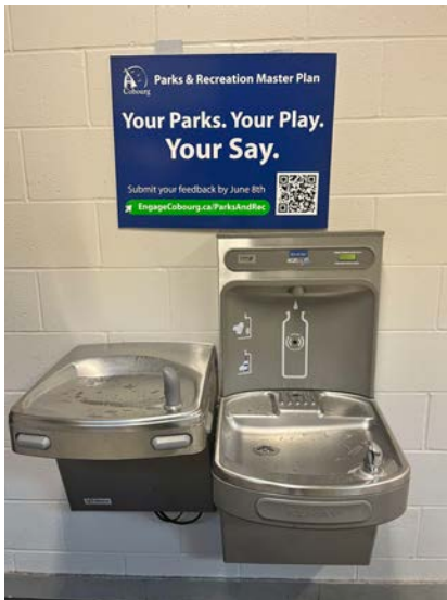
Figure 2.7: Drinking Water Fountain and Bottle Filler inside the CCC
