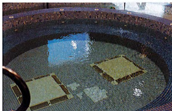
Photo 26: Pool Basin - Entrapment Cover
