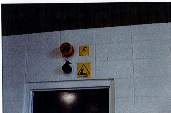
Photo 33: Carbon Dioxide Alarm
