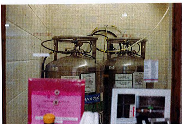
Photo 35: Carbon Dioxide Tanks
