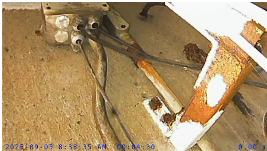
Junction box to be replaced and relocated
