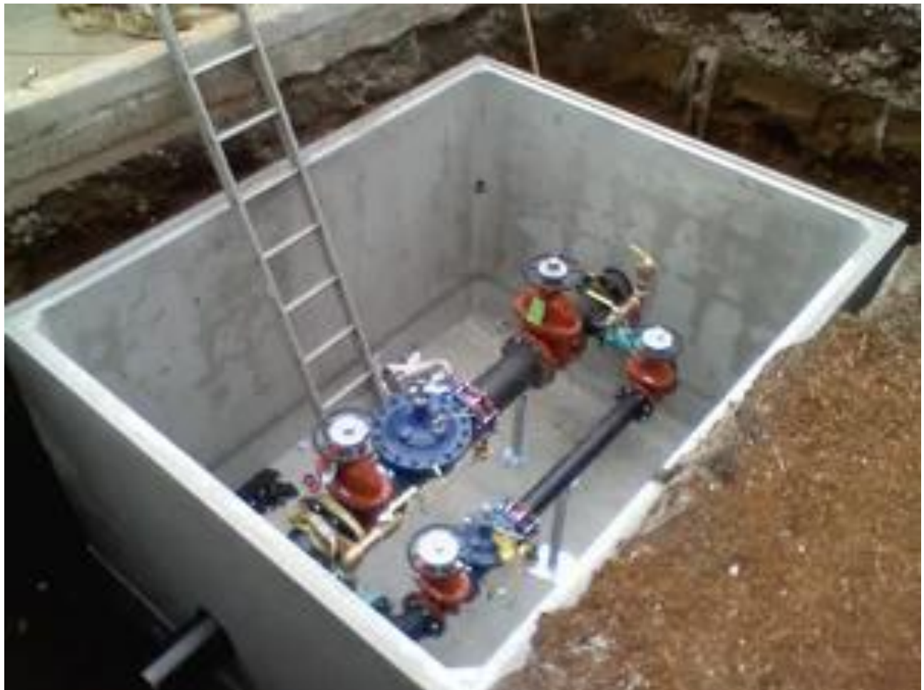
Meter Vault Example
