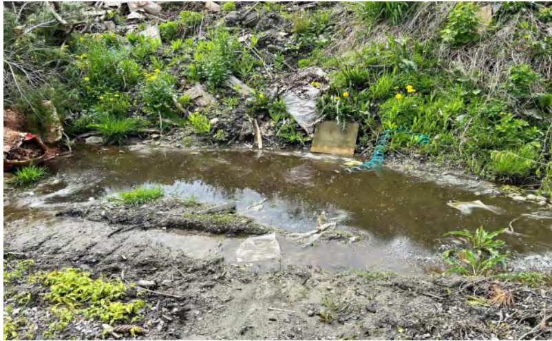
5. Ponded water in fill area. (May 2024)
