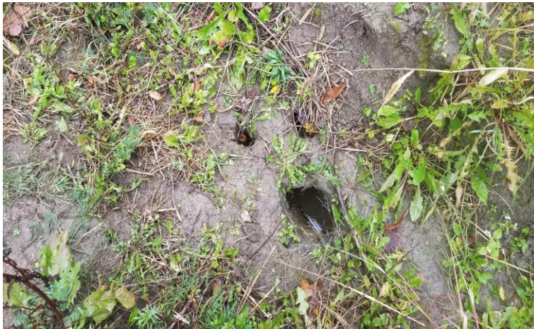
11. Hickenbottom® Drain Outlet. (October 2023)
