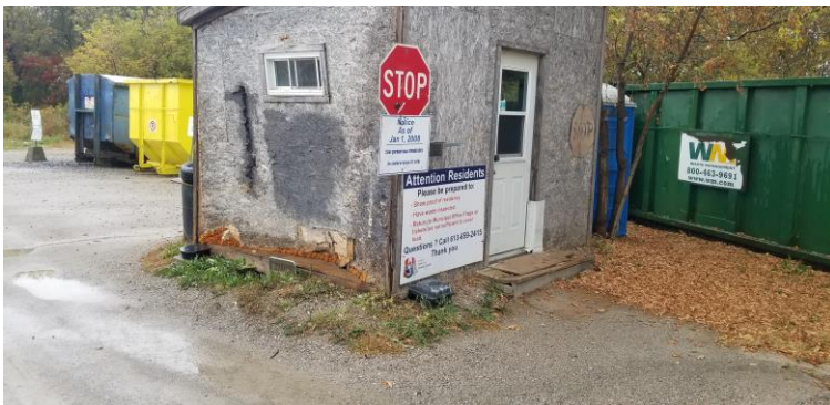
11. Attendant shed deteriorating on left side. (October 2023)
