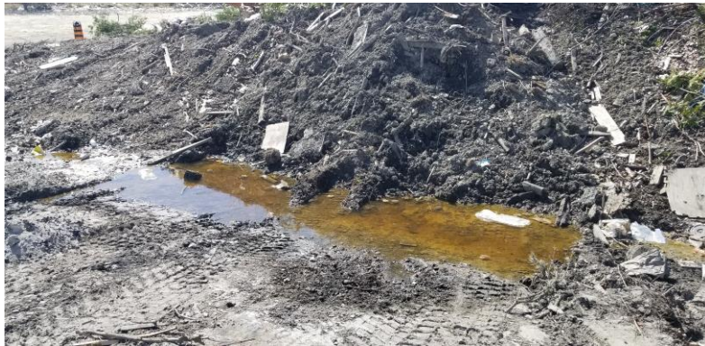
1. Ponded water in fill area. (April 2023)
