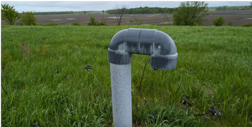
Photo 7: Vent on the capped waste mound.
