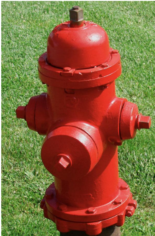
Figure 18. Example of a private fire hydrant.
