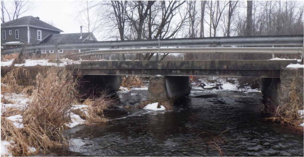
Figure 3-1: Example of Poor Condition Bridge or Culvert – Donovan Bridge
