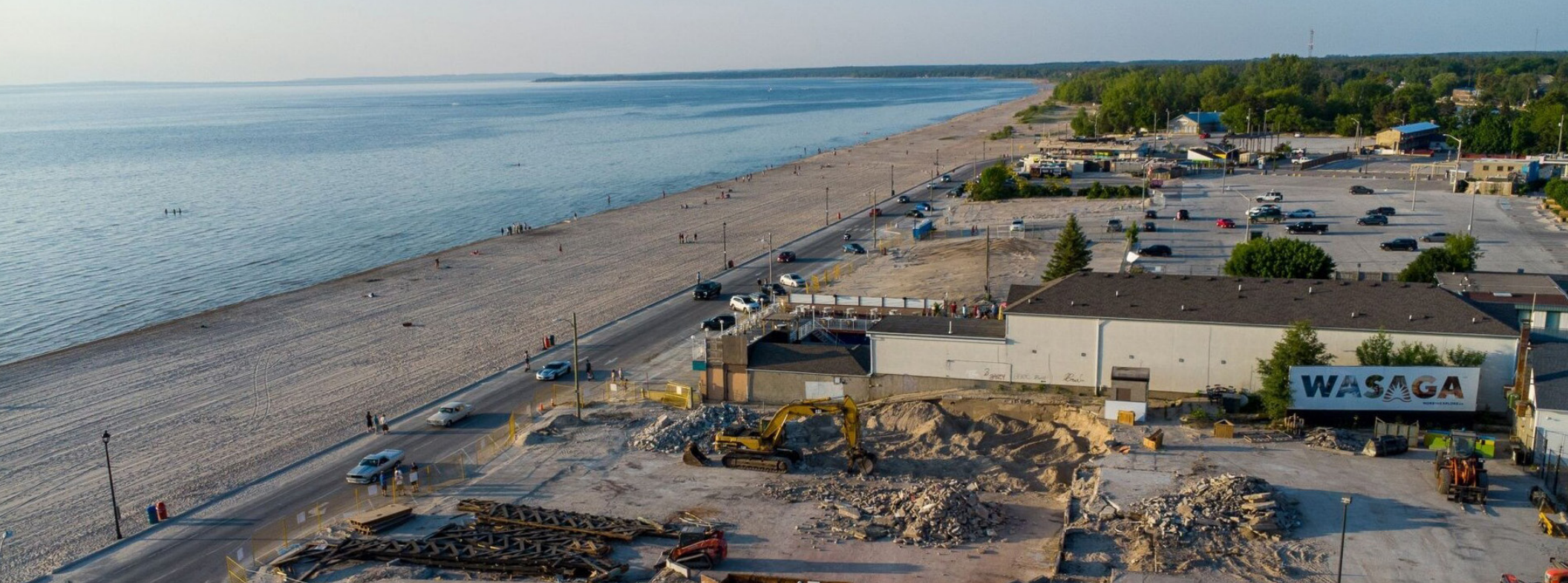
Fig 24. A 2007 fire destroyed several buildings at the Main End. In 2015, the Town purchased a number of aging seasonal commercial properties that had suffered repeated flood damage and were not built for year-round use. In 2025, the buildings were demolished in preparation for the reconstruction of Beach Drive and future development.
